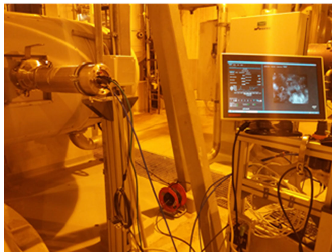
Figure 2: Bubble size measurement system installed in the process, including on-site control and monitoring capabilities
