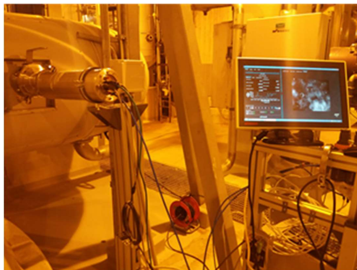
Figure 2: Bubble size measurement system installed in the process, including on-site control and monitoring capabilities
