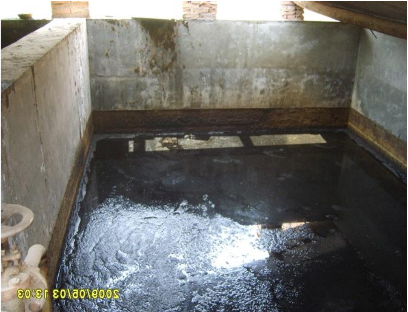
PICTURE 1. Waste oil storage tank. (adapted from Yao 2010.)
