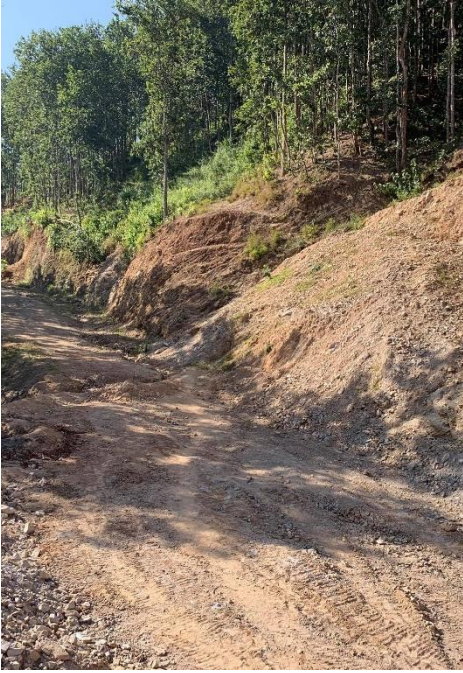
Figure 1. Condition of the gravel road before the upgrading project
