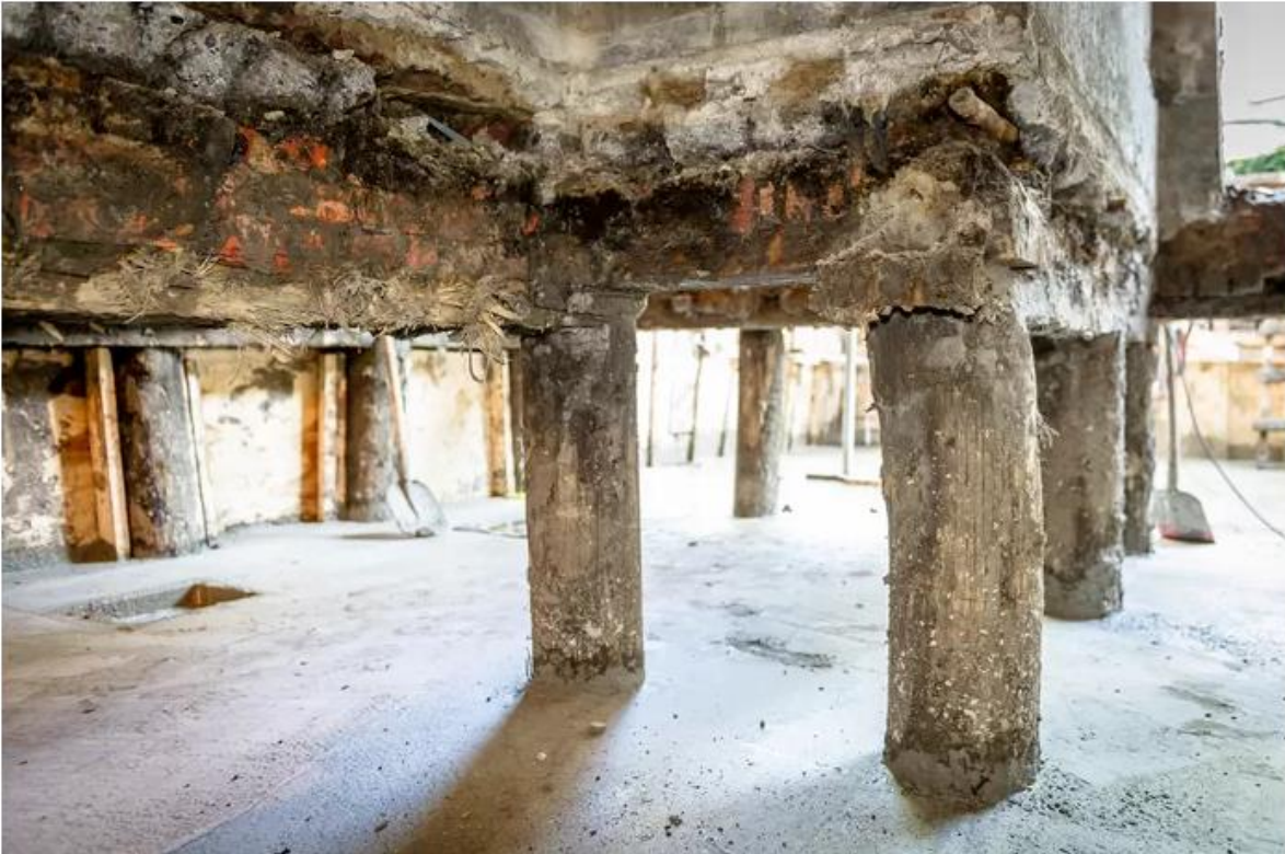
Figure 13 Photo of a rotten exposed wooden foundation in need of repair (Algemeen Dagblad, 2020)
