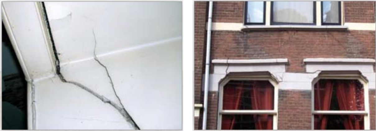
Figure 11 Pictures showing cracks on the inside and outside of the building (VROM, n.d.)
