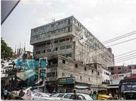
FIGURE 18: Rana Plaza before collapse (Source: Wikimedia Commons, 2015)
