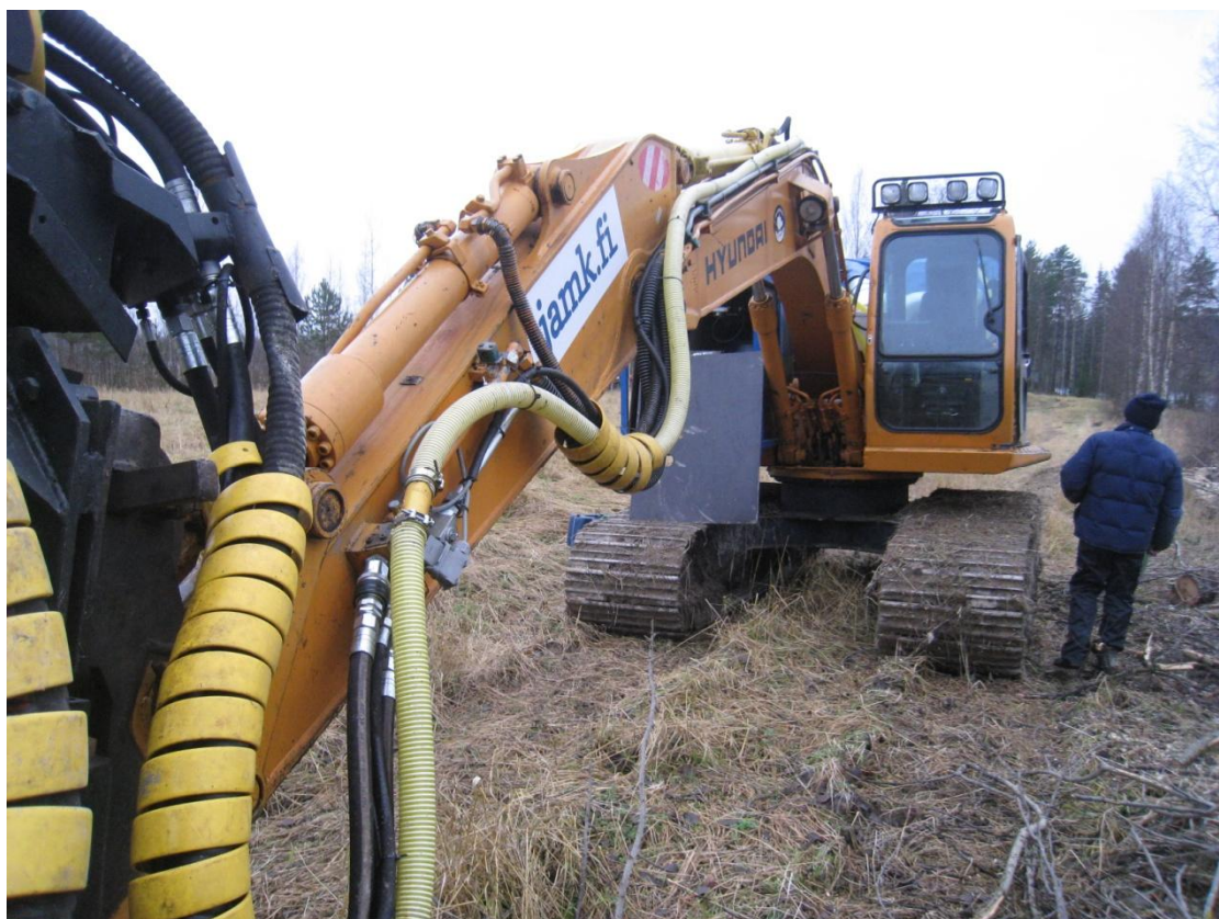
FIGURE 11. Sawdust goes through the pipes.
