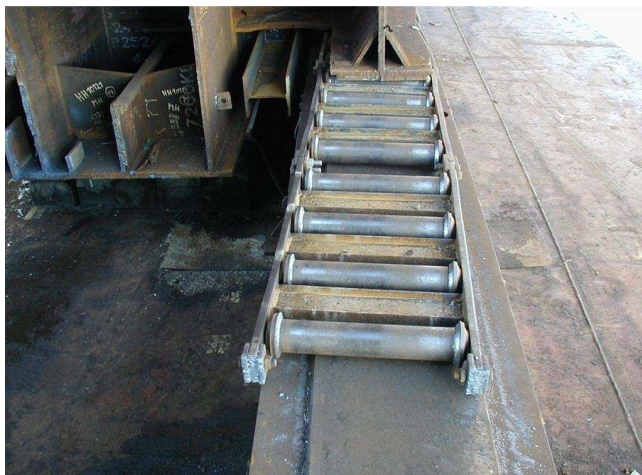
Figure 2.2.3: Roller unit out of line
