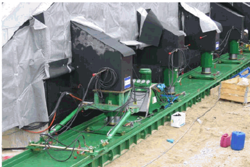
Figure 4.2.2: APS-system in use. /10/
