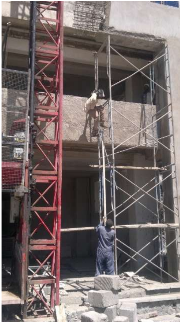
Picture 1. Workers at risk when transporting goods.
