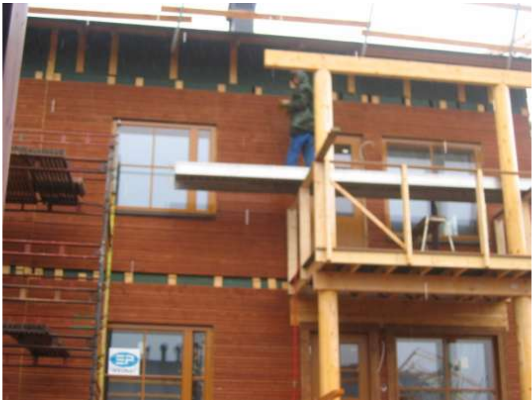
Picture 3. Work on a dangerous base.
