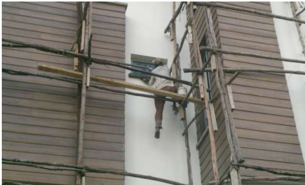
Picture 2. Working at height without a harness on Kenyan site.
