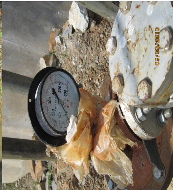
Photo 4: Broken meter need to be changed
