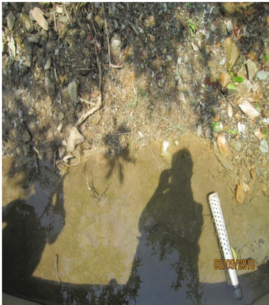
Photo3: Debris inside intake, cleaning and slab needed changed
