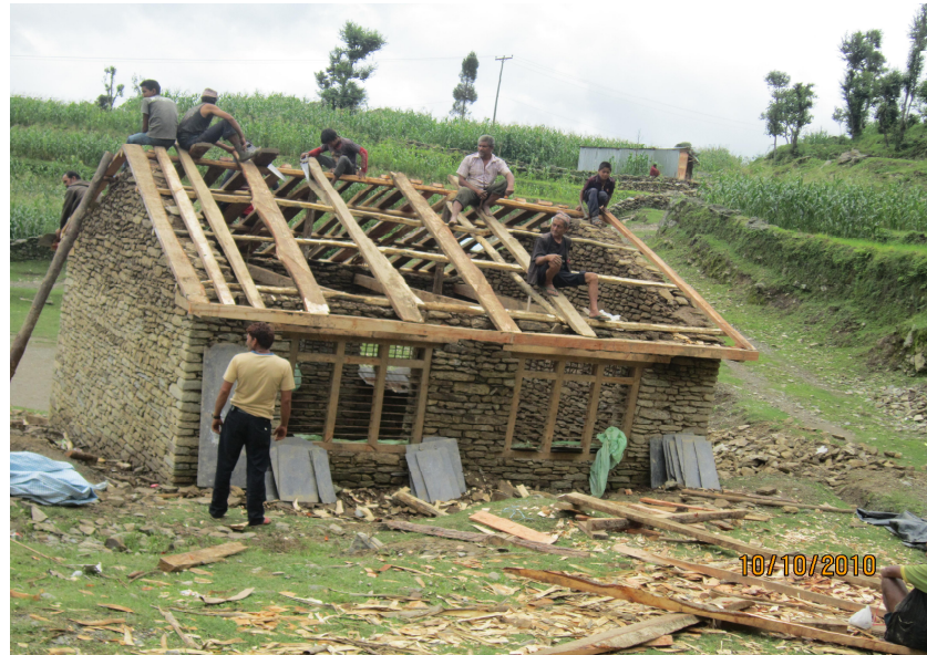
Photo 6: After completion of water scheme users' are involved in the Construction of community building using the same modality
