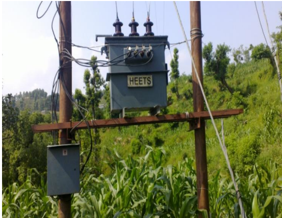
Photo 1: view of transformer fencing needed
