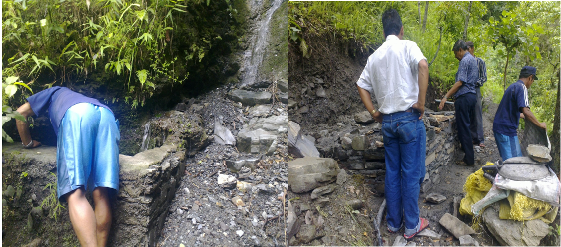
Photo 1: Source Tapping Point near landslide area construction, sliding area observed
