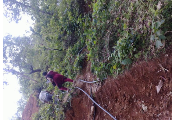
Photo 5 and 6: Open pipelines at different stretches in distribution system need to be buried at proper depth
