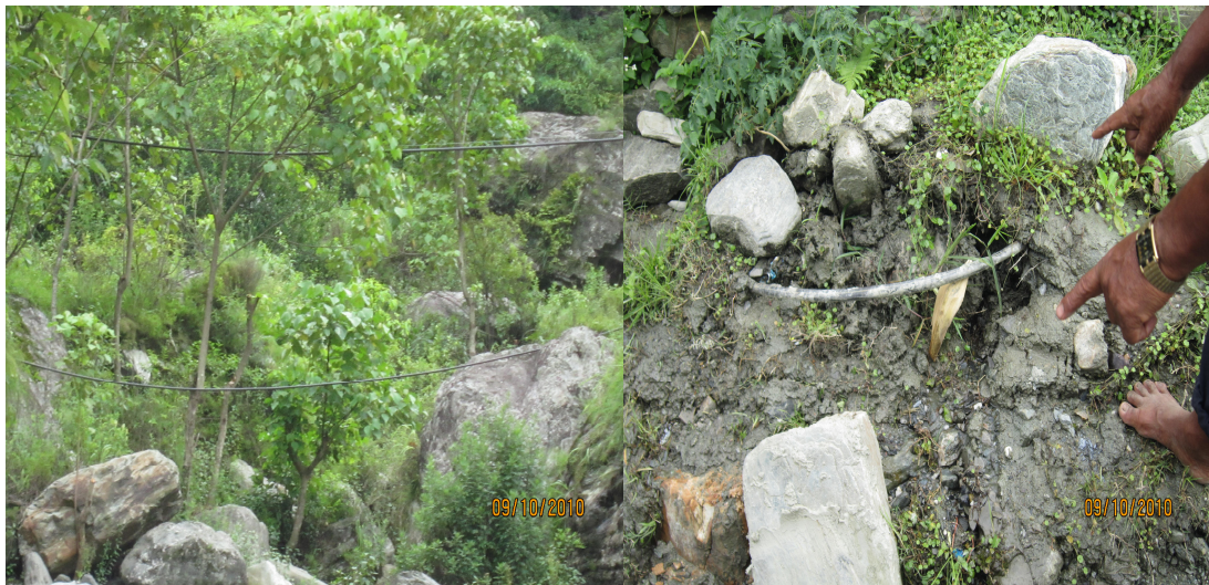
Photo 5: HDP pipe at crossing, needs proper support village road; to be properly covered
