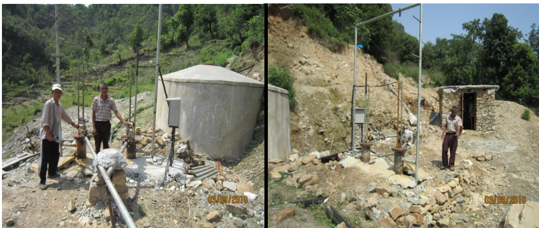
Photo 5: 1 st pumping station, site clearance and fencing needed due to road construction; protection measure needed.
