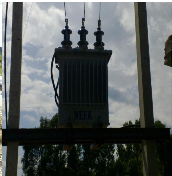
Photo 2: Transformer for the scheme
