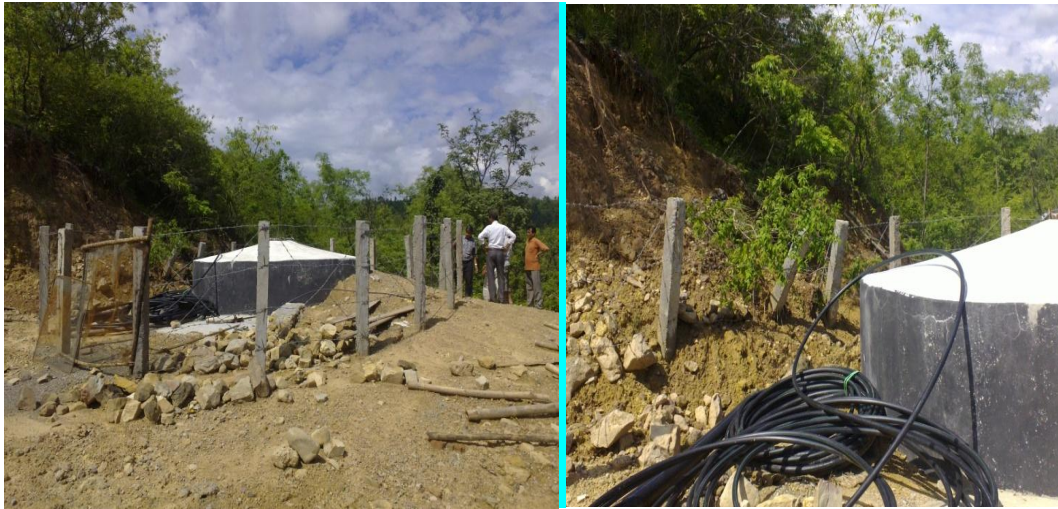
Photo 3:- RVT good workmanship; site clearance and backfilling left Photo 4: Fencing improvement at north part with protection work (masonry wall) needed to stop sliding.
