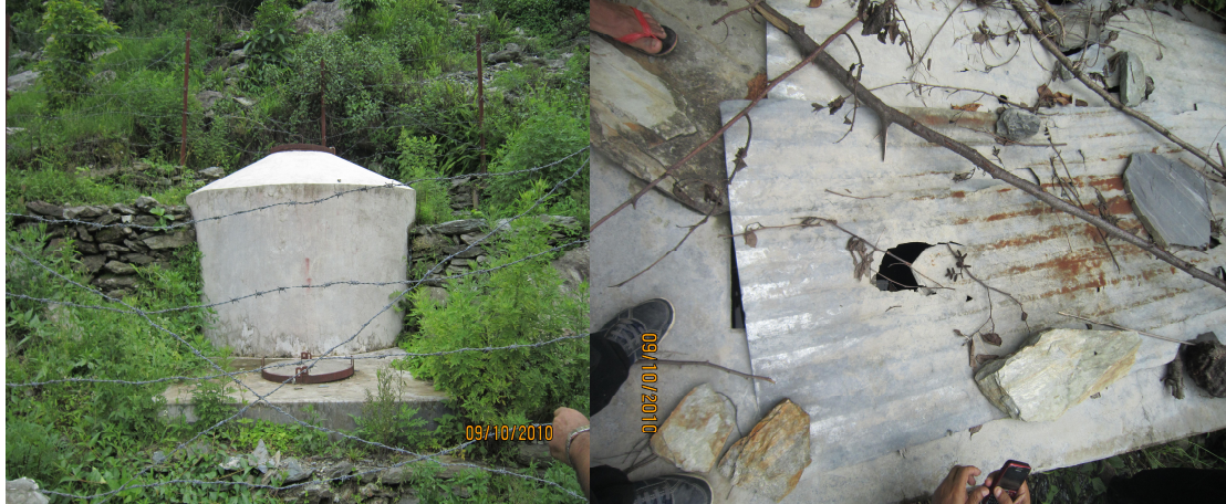
Photo 3: View of RVT; regular cleaning needed cover; need to be changed
