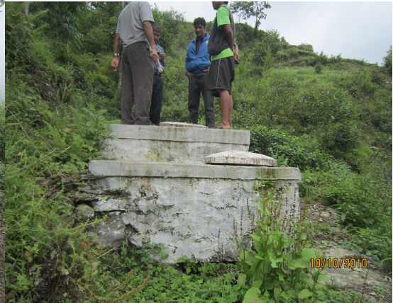
Photo 4: View of RVT; cleaning work needed
