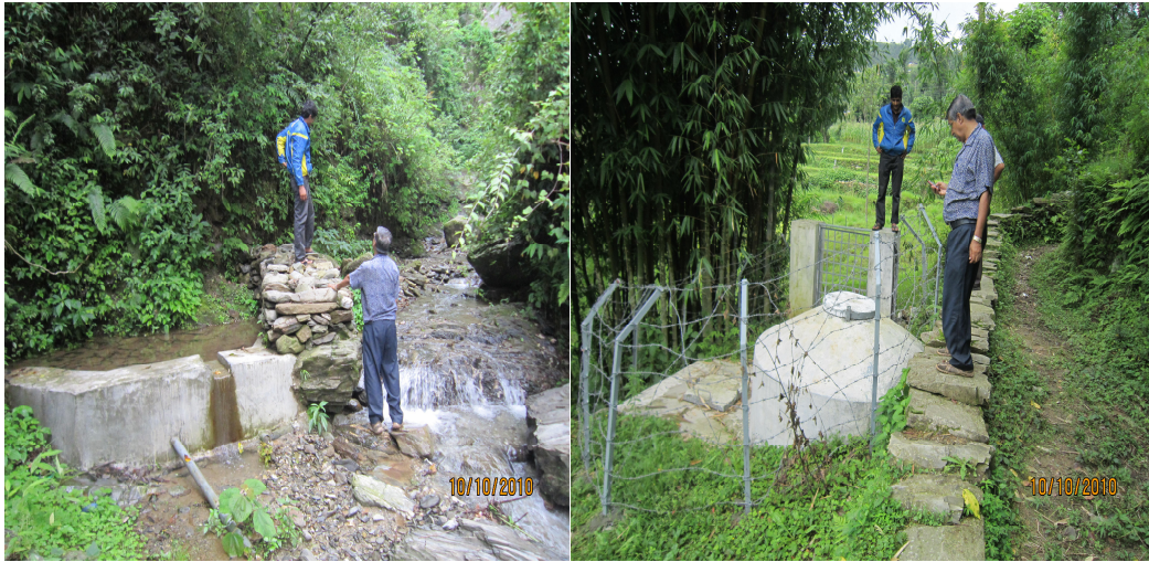
Photo 1: View of 1 st Intake and catchment Area good construction quality and fencing
