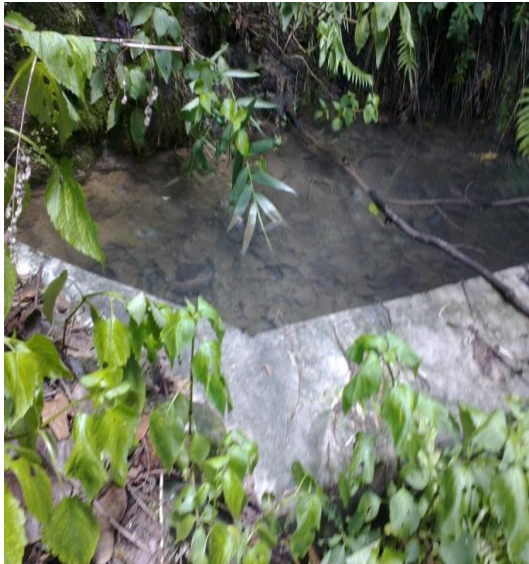
Photo 1: - Intake structure; needs proper cleaning cleaning and fencing
