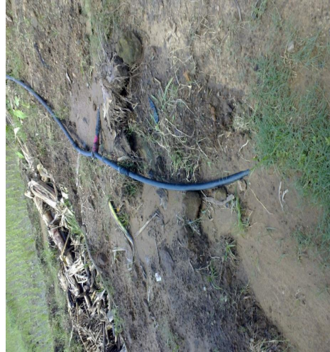
Photo 5 and 6: Pipelines not buried properly as the users cut and thrash it from time to time to remove lime;
