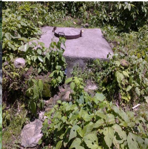
Photo 2: - collection chamber needs proper
