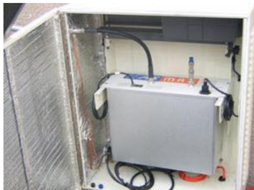
Figure 8. A WiMAX radio placed inside an enclosure box for safety.
