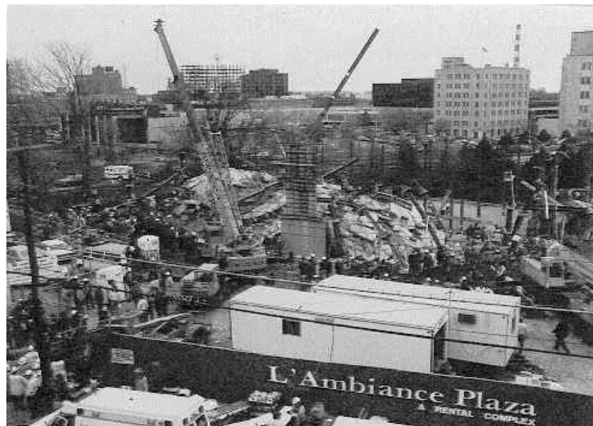
Figure 4. Failure of L'Ambiance Plaza under construction
