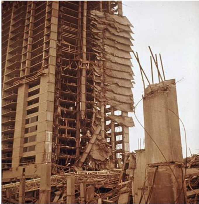
Figure 2. Skyline Plaza, 1973 – premature formwork removal
