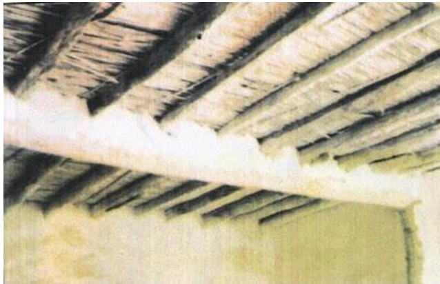
GRAPH 12 Poorly made roof of an Egyptian rural house (adapted from http://mirathlibya.blogspot.fi/2010_02_01_archive.html )
