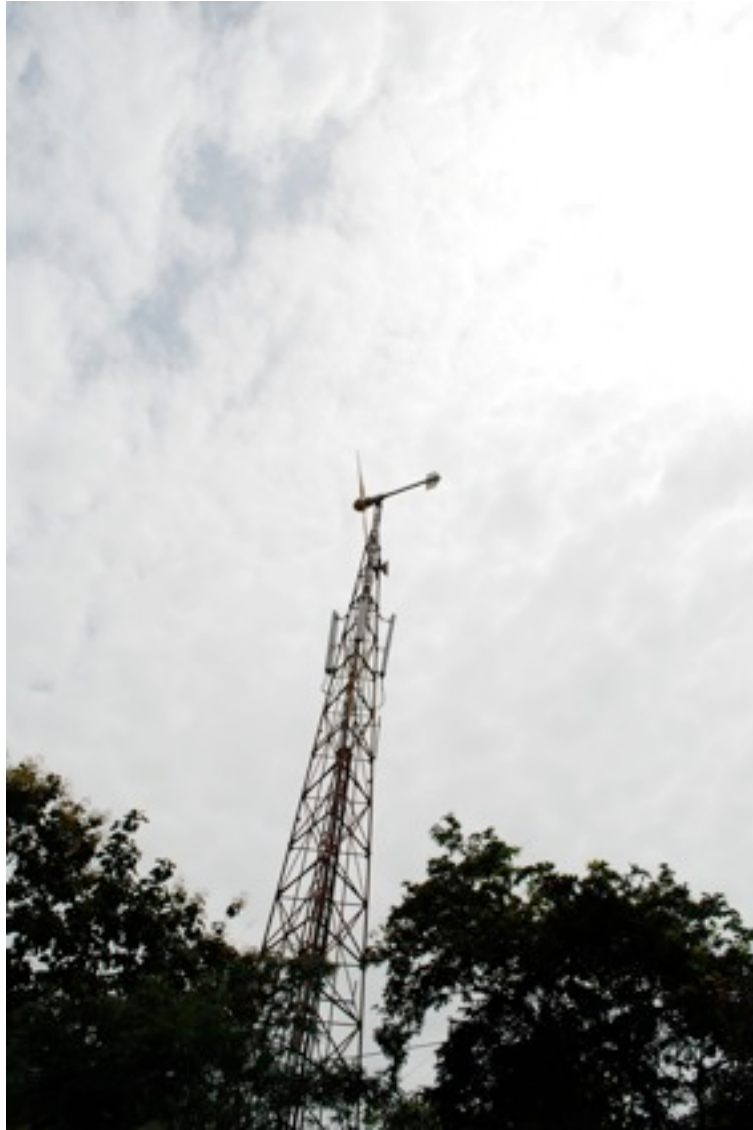
Figure 17. Windmill powering a telecommunication tower in Alibag, Maharashtra state. (Picture by Manoj Roy)
