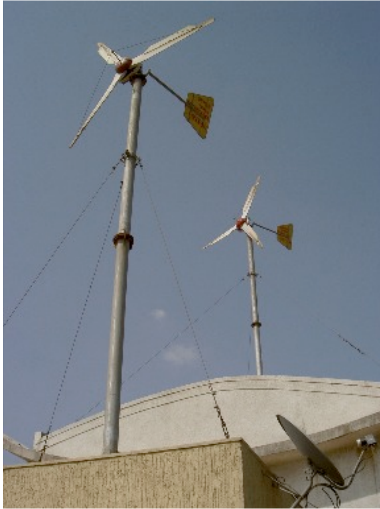
Figure 10. Supernova Technologies's 1,4 kW wind turbines on the top of the Lords Building in Navi Mumbai. (Picture by the author)
