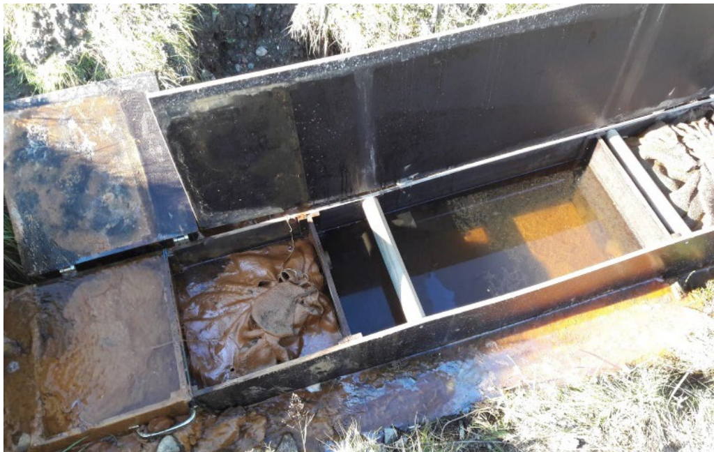
Figure 3. The passive barrier filtration system installed in runoff outlet point in Kajaani.
