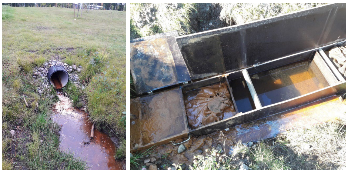
Figure 2-3: Contaminated runoff water outlet and PBS. (Photo: Kai Tiihonen)
