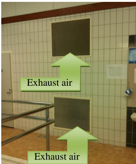
FIGURE 21. Exhaust grids in the interior wall
