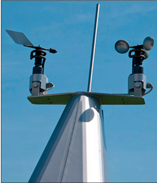
Figure 3.20. Measurement sensors of wind direction and wind speed in a nacelle.
