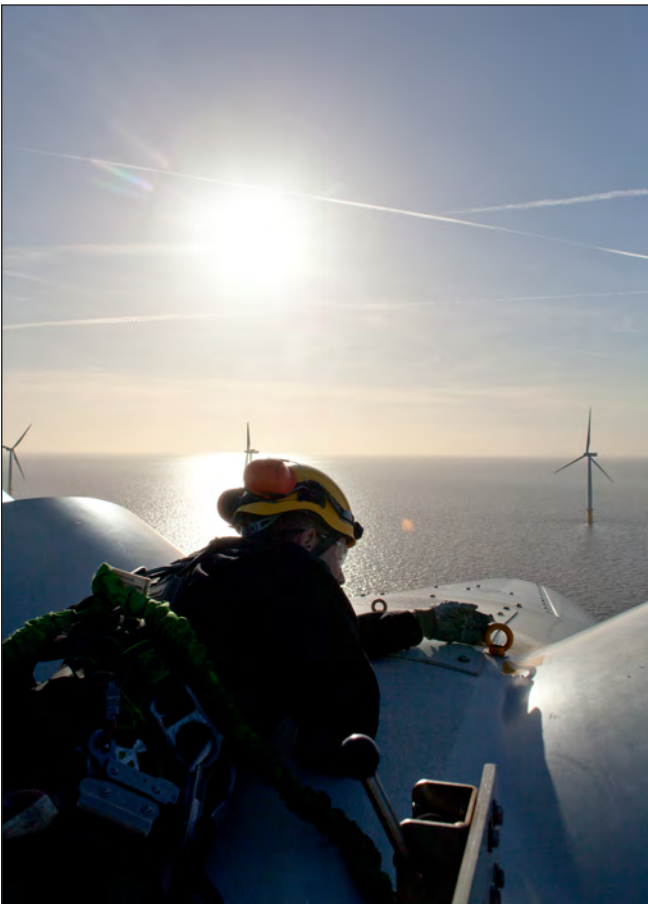
Figure 4.4 Well-planned maintenance operations required on land and at sea (Siemens Press Pictures 2013)
