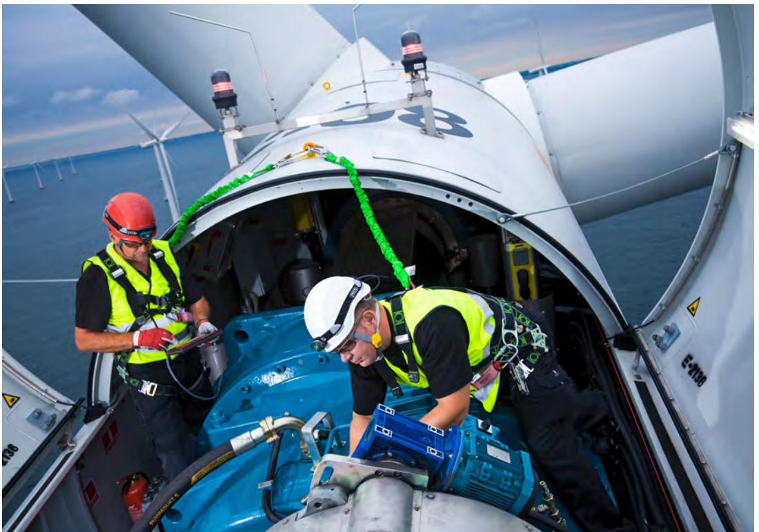
Figure 4.1. Two Siemens service engineers working in the nacelle of a wind turbine at Sweden's Lillgrund offshore wind farm (Siemens Press Pictures 2008)
