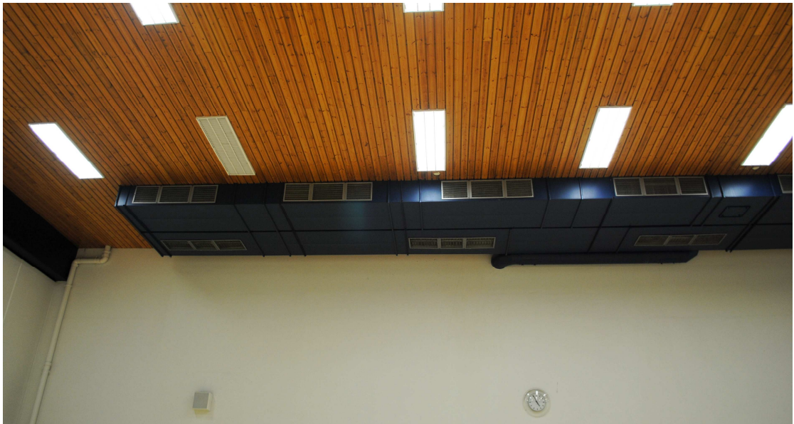
FIGURE 11. Ventilation and Air-conditioning system in the sport hall
