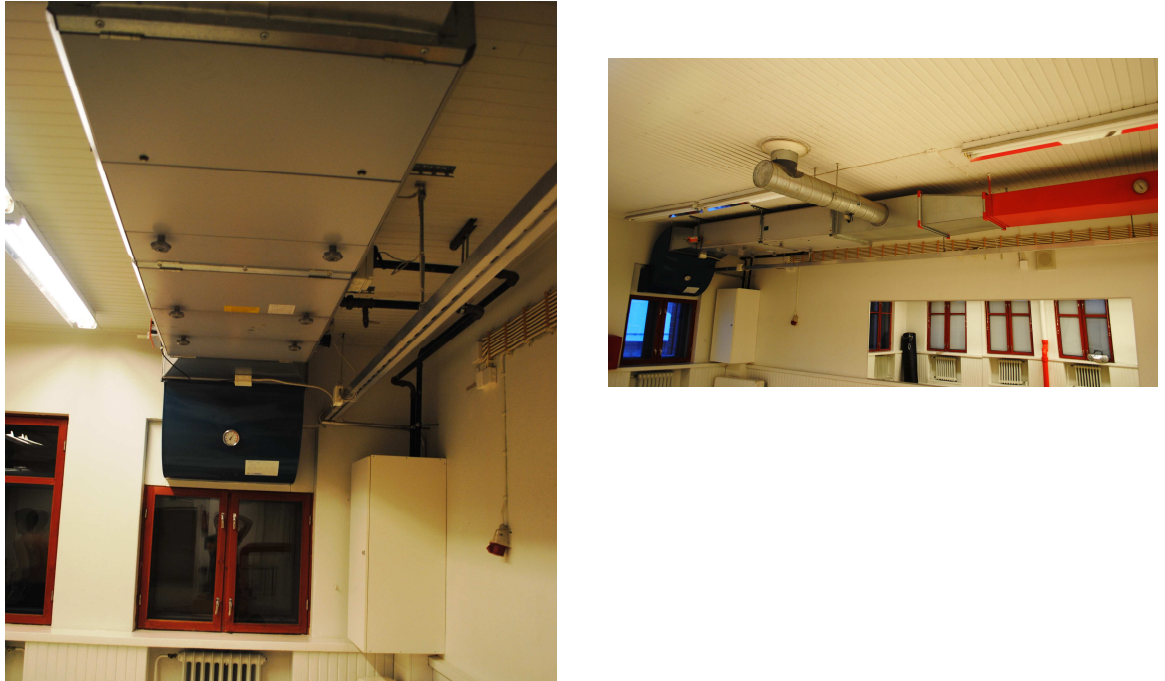
FIGURE 29. Mechanical ventilation in gym
