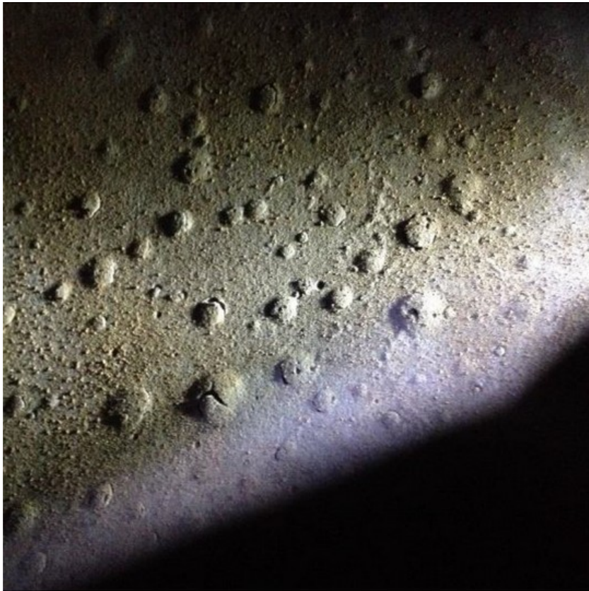
Figure 9. Hydrogen blistering in an amine absorber column. (Gregory N. Haidemenpoulos etc. 2018.)
