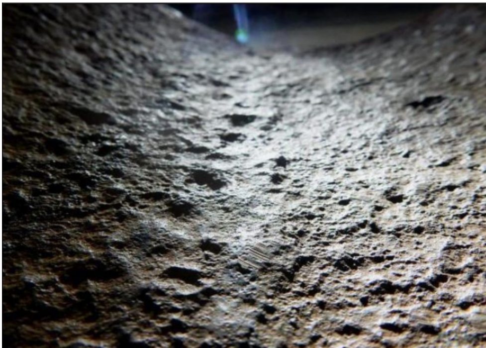
Figure 7. Close view of the internal surface of a suction header corroded by sour water. (Manoj Kumar etc. 2017.)
