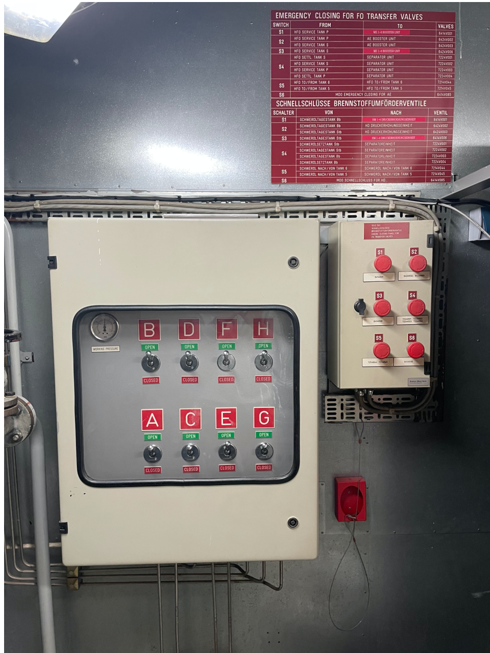
Figure 21 Safety station fuel valve emergency closing unit (Alo Kask, 2022)
