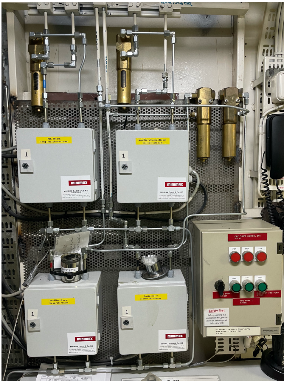
Figure 20 Safety station CO2 system release (Alo Kask, 2022)
