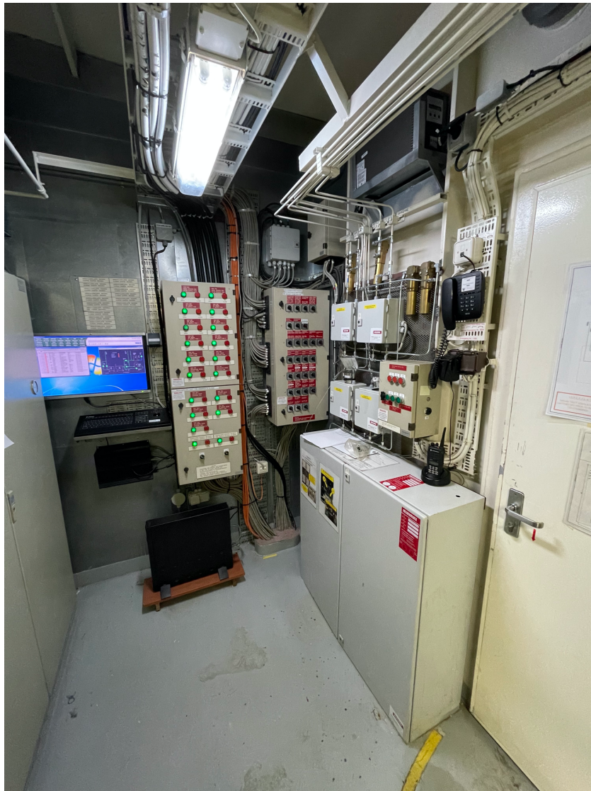
Figure 19 Safety station (Alo Kask, 2022)
