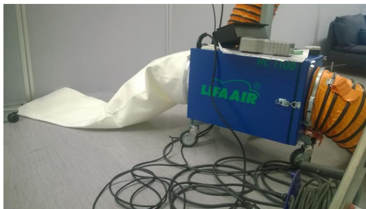
Figure 11. On final stage the F7 class exhaust filter was added to negative pressure unit.
