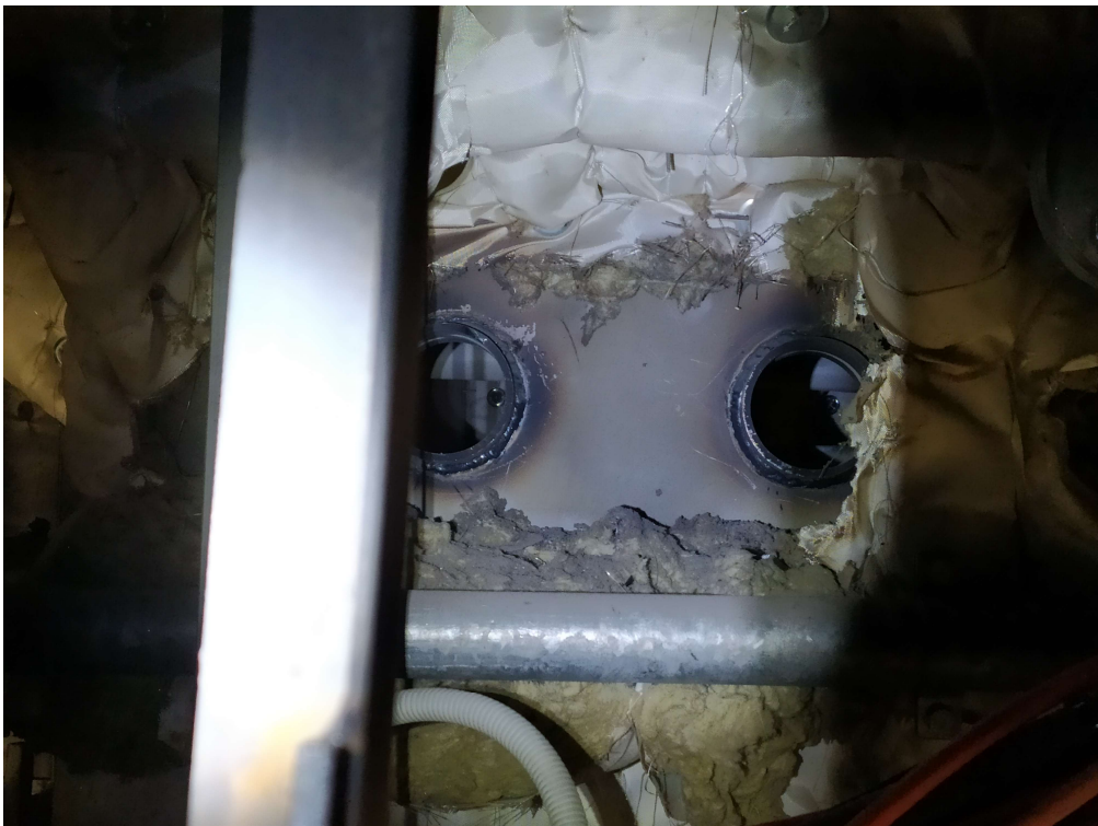
Figure 21: Damaged insulation. Penetrations not done in proper stage result in additional works to restore condition of finished technical area. Penetrations need to be cleaned, coated and re-insulated.
