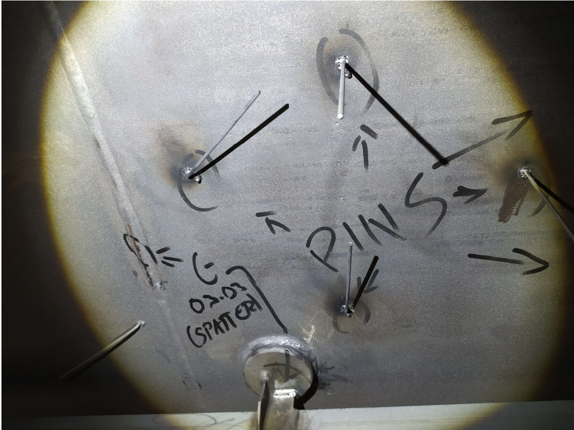
Figure 18: Missing insulation pins discovered by author during inspection re-installed. Note welding dust not cleaned after re-instalment of pins.
