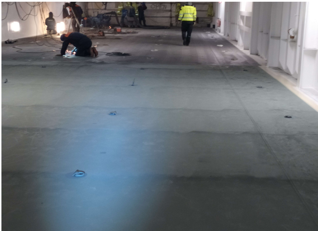
Figure 4: Zinc based stand-alone coat on car deck. Metalworks on-going on background. Note that the zinc coat has been sprayed poorly resulting excess or low DFT on overlapping areas. Based on 80-20 principle the area was accepted.
