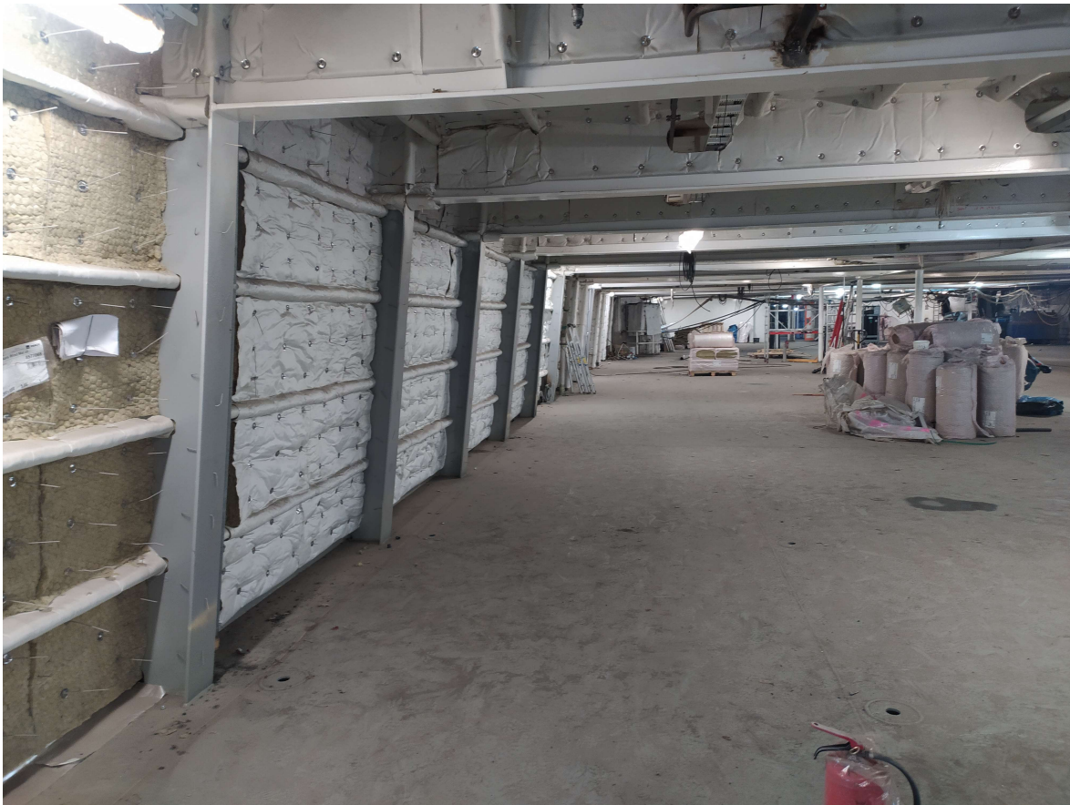
Figure 16: Fire- and thermal insulation. Thermal insulation placed on top of fire insulation as additional layer on ships cargo area on outer bulkhead insulation.
