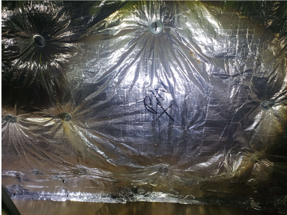
Figure 19: Missing insulation pin discovered by author during inspection of insulation.
