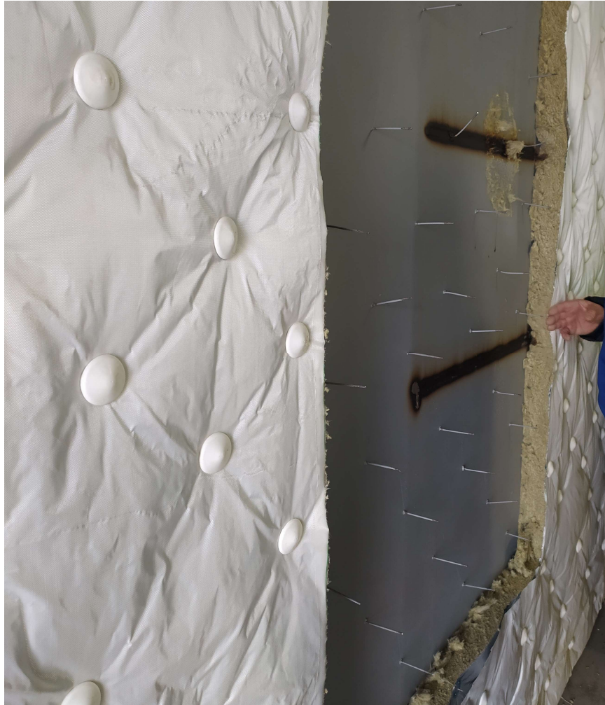
Figure 17: Insulation caps used to prevent injuries.
