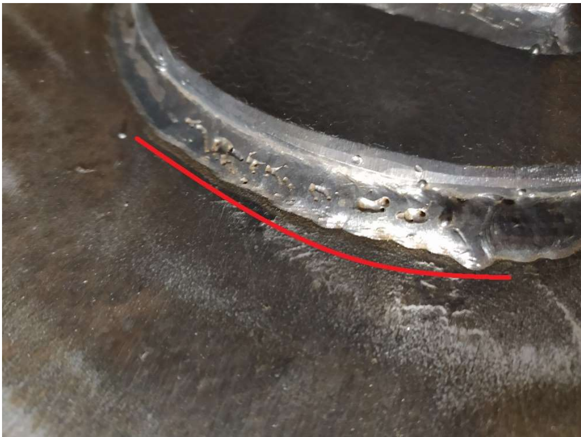
Figure 7: Example of poor welding quality. Pinholes and weld-spatter revealed on wire-brushed area.
