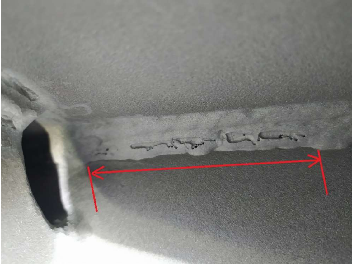
Figure 6: Example of poor welding quality. Pinholes revealed on freshly blasted area.
