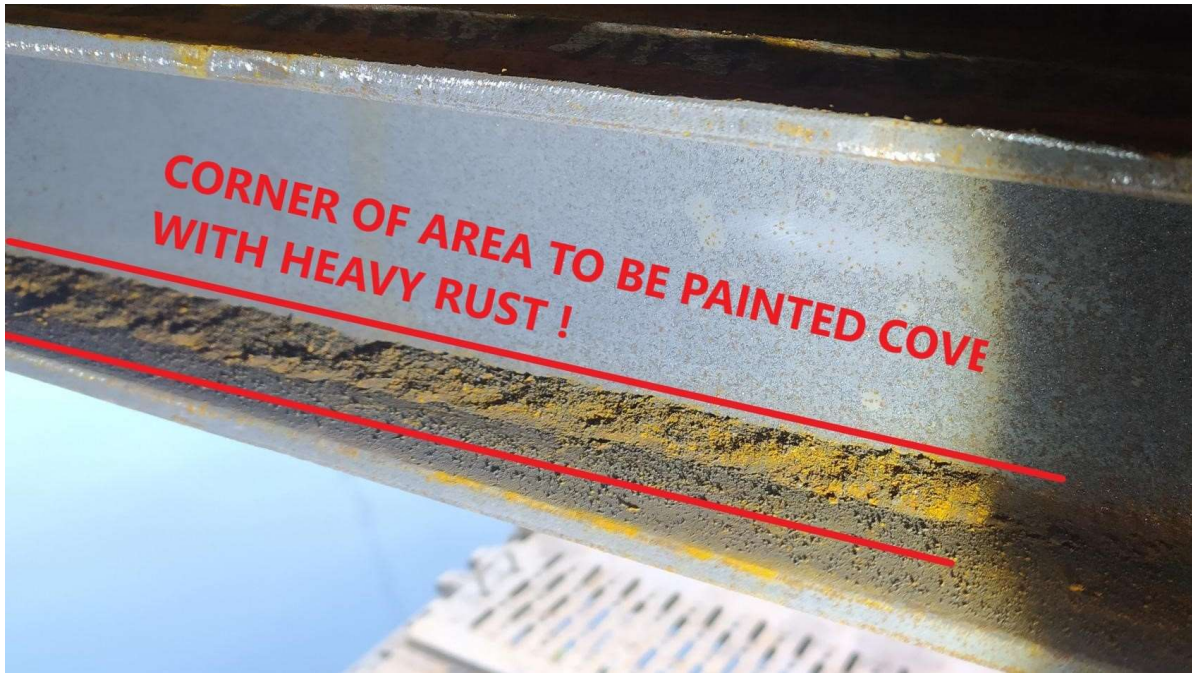
Figure 8: Area covered with heavy rust found during metal inspection prior painting.
