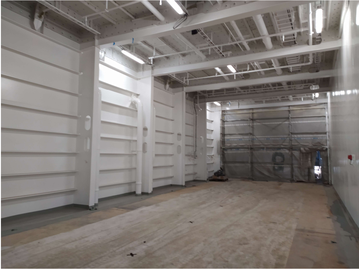
Figure 13: Final layer bulkheads and ceiling on cargo area. Ceiling insulated with fire insulation. Deck level still to be blasted and coated.
