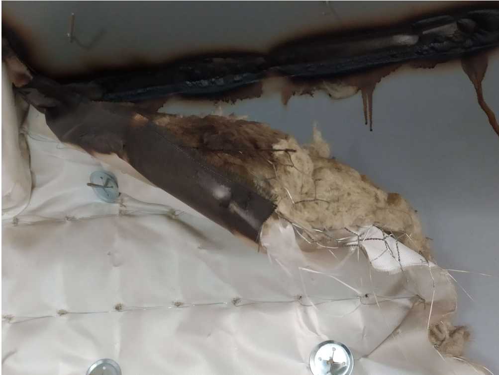
Figure 20: Damaged insulation after apparent welding on upper deck. The metal surface should be cleaned, re-coated and re-insulated.
