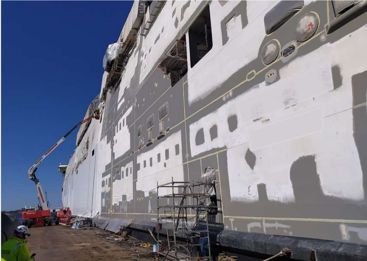
Figure 3: Side shell painting. Painting done in sectors. Area in background covered with top-layer while the aft area is stripe-coated. final inspection prior topcoat carried out. Note that filler has been used and left uncovered by primer on various spots on aft sector and the sector was not approved for top-layer painting.
