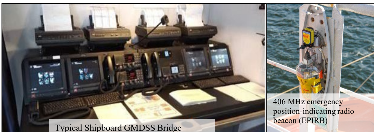
Figure 2 Ship Bridge GMDSS Installation and Float Free EPIRB
