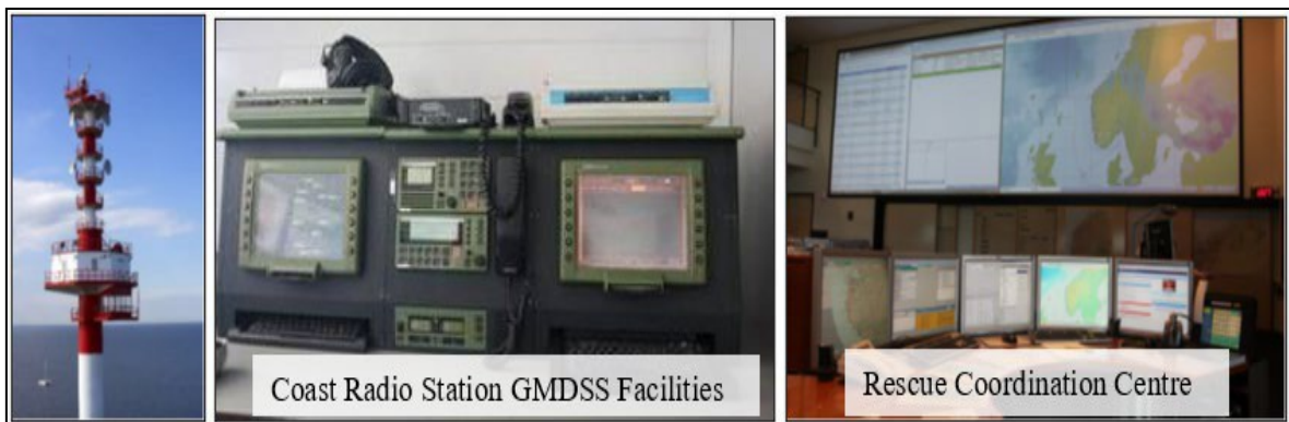
Figure 3 Typical Shore-side GMDSS Infrastructure and Rescue Coordination Facilities
