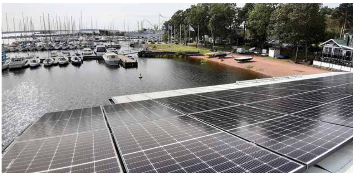
Picture 5. New solar power plant in Sapokka small port in Kotka, Finland.
