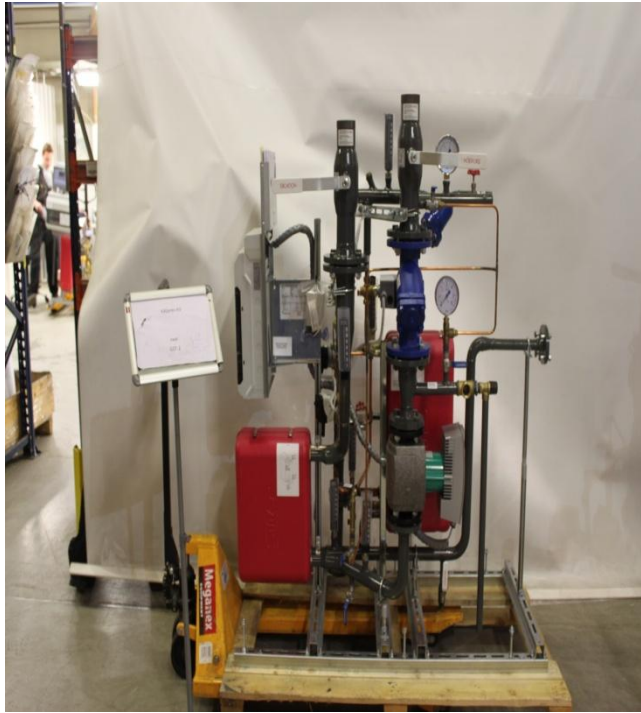
FIGURE 5. Parallel coupling heating substation, horizontal structure, DN 65, four-point measurement in heating secondary side, safety valve, thermometers, gauge block for energy meter and pressure gauge in DH Return, two point measurement in DH Supply
