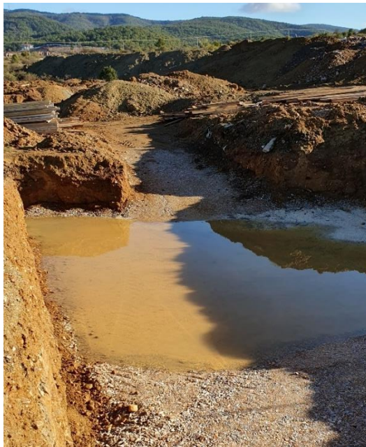
Figure 1 Foundation filled with gravel flooded by rising of water from water capillaries
