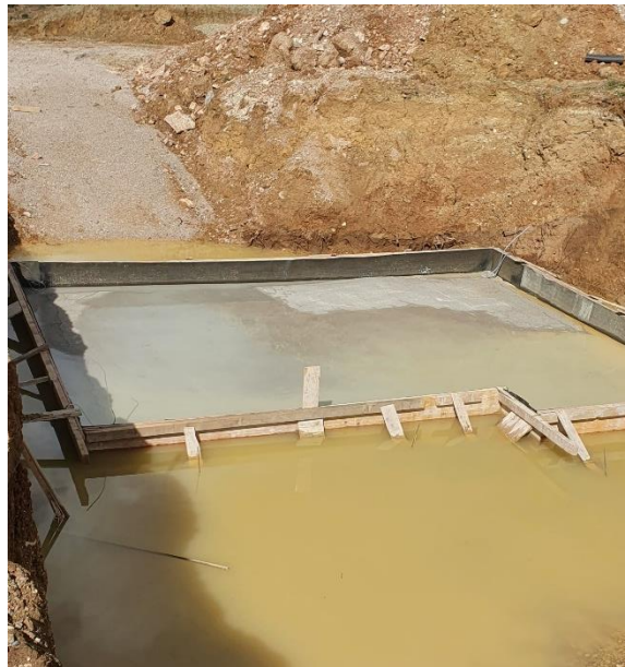
Figure 2 Highly damaged concrete slab used for foundation from heavy rain
