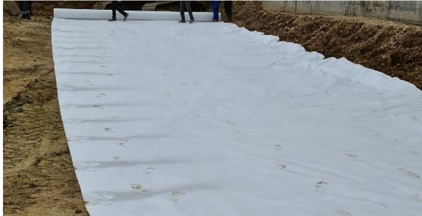
Figure 5 Geotextile layer (5 mm) being applied to prevent water rising through the gravel for the foundation of a residential 8-story building
