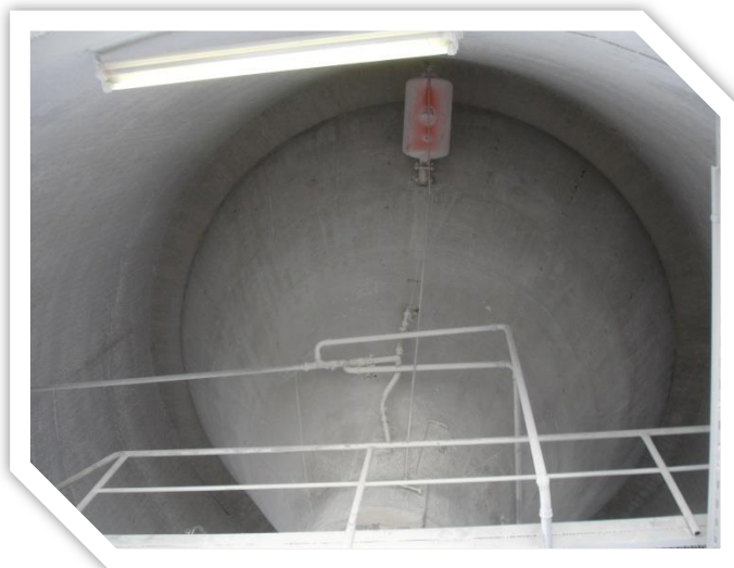
Figure 15 Air-cannon in limestone discharge silo.
