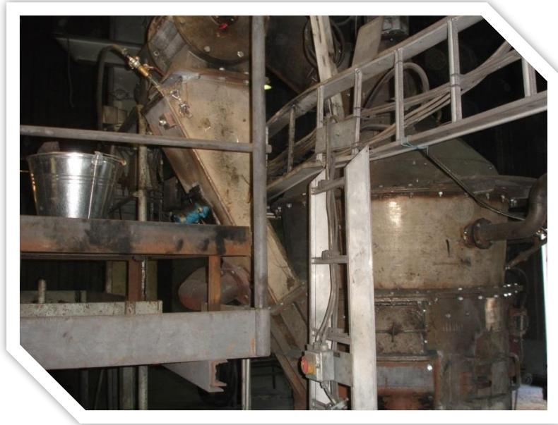
Figure 14 Coal feeding chute. Nordkalk Oy.
