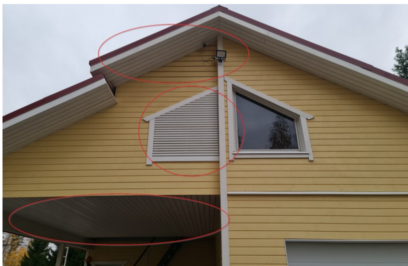
Figure 22. The "ventilation" of the panels (Niskala 2022)
