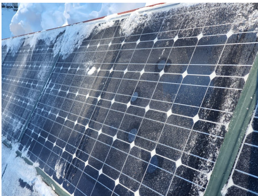
Figure 56. Defective panels in action (Niskala 2022)
