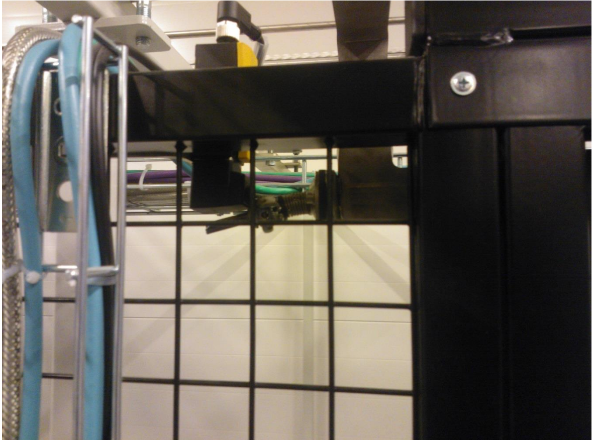
Figure 21 Safety switch's actuator does not always hit to the right place.
