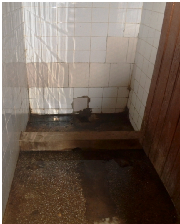
FIGURE 15. "Drain urinal" for female users in Ho Central Market
