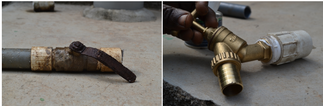
FIGURE 11. On the left, the old rusted valve and on the right, the new more suitable valve
