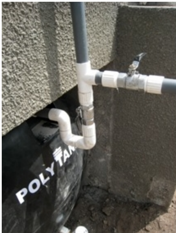
FIGURE 10. Urine tanks' cleaning valve (Aalto etc. 2012, Annex 8)
