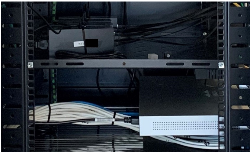
Figure 12. PoE adapters mounted in rack cabinet above switch.
