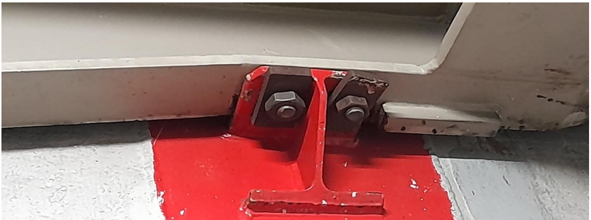
Figure 25: Bolts that securing the tween deck.
