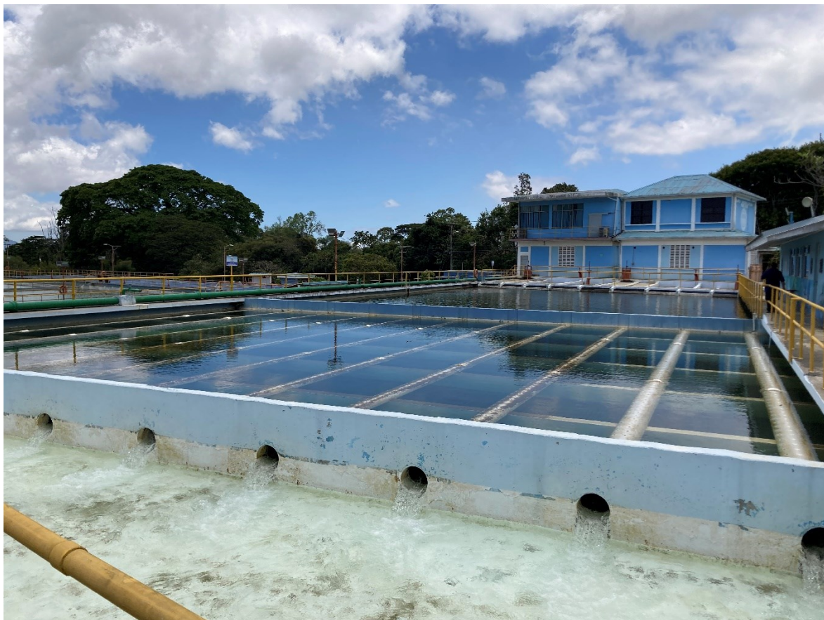
FIGURE 3. Laminated sedimentation basin at Tres Ríos water treatment plant (Hoffrén 2023, CC BY-NC)
