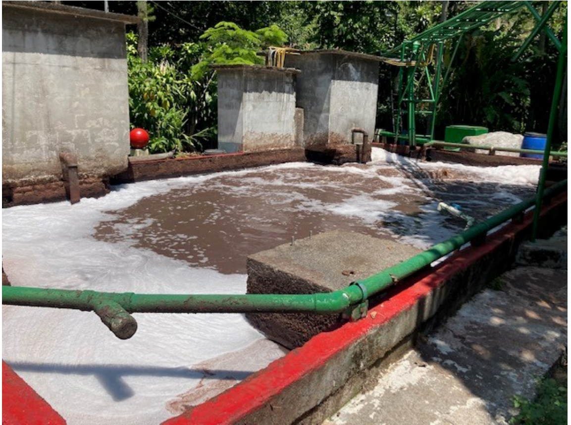
FIGURE 14. Tenería Pirro's biological treatment process (Hoffrén 2023, CC BY-NC)
