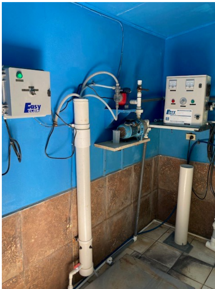
FIGURE 6. Disinfection pumping system at ASADA Santa Elena (Hoffrén 2023, CC BY-NC)
