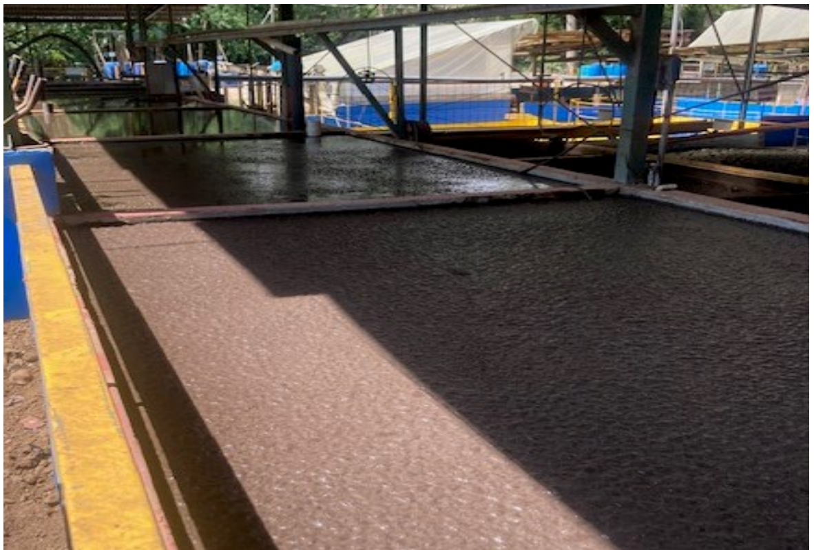
FIGURE 12. Biological treatment basins at Fumigadora Alto (Hoffrén 2023, CC BY-NC)
