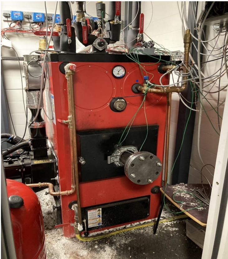
Figure 6. Veto-60 Kw biomass boiler
