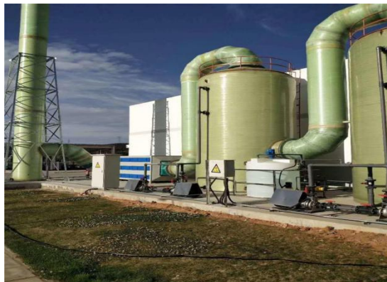
(2.3.1) The denitrification tower system
