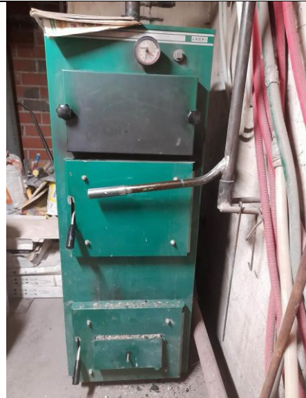
FIGURE 5. The building wood boiler.
