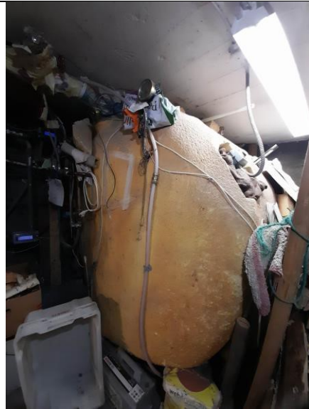
FIGURE 4. The building hot water tank covered by insulation.
