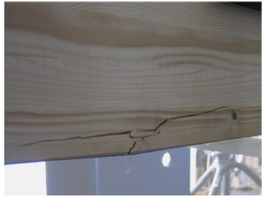
Fig. 7. Tension failure under bending.
