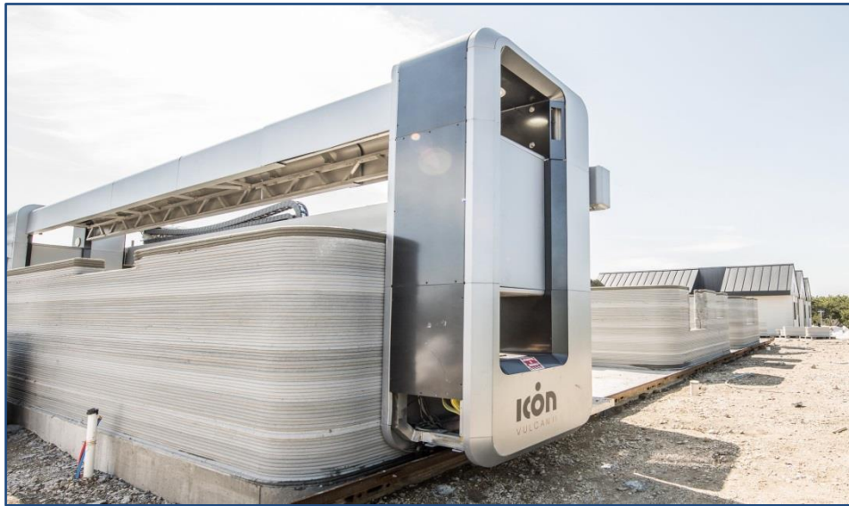
Fig. 22 Vulcan 1 Printer by ICON is a gantry system printer used for building small size family homes in Mexico 30
