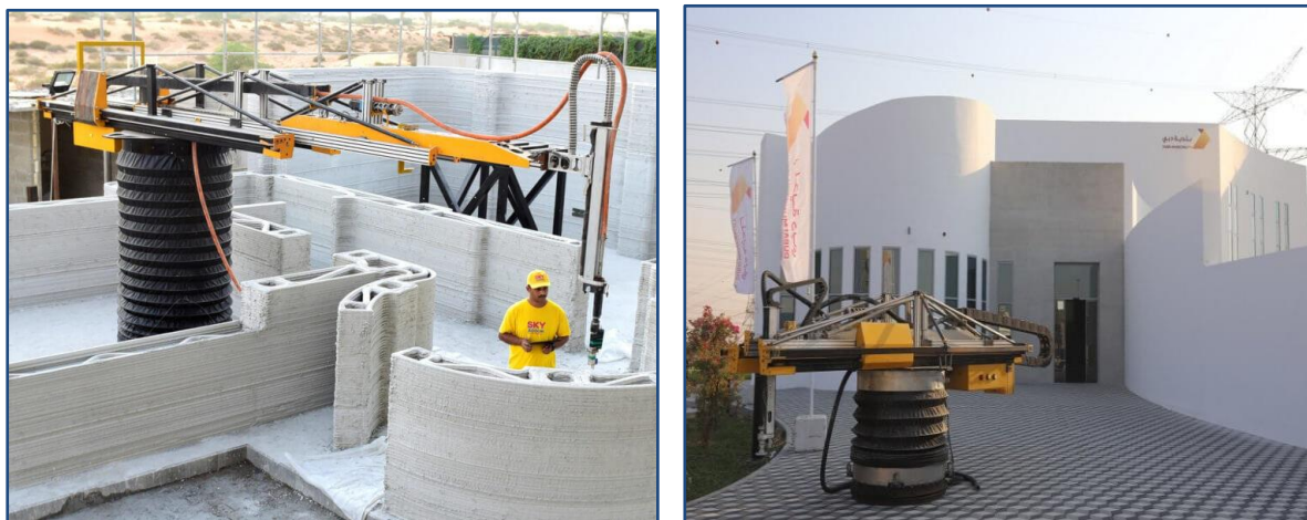
Fig. 25 Left: Apis Cor Robotic arm printing system at work. Right: The completed printed building
