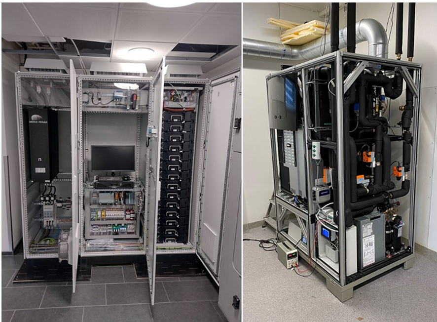
Fig. 3 92 kWh battery energy storage (left) and heat pump integrated 15 kWh latent heat storage (right) installed in target building at Tampere University of Technology
