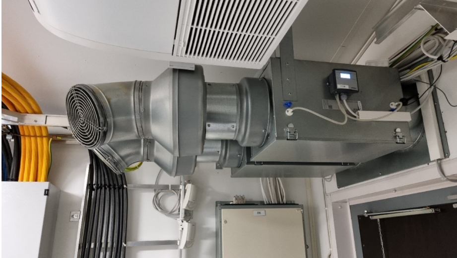
Figure 7 DC fans installed as an emergency cooling device
