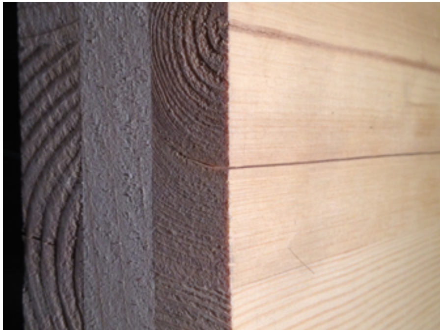
Figure 8. Deep cracks in 60mm three layered CLT
