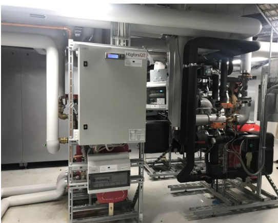
District Heating Substation
