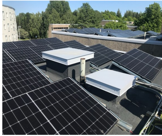
Photovoltaic solar panel system
