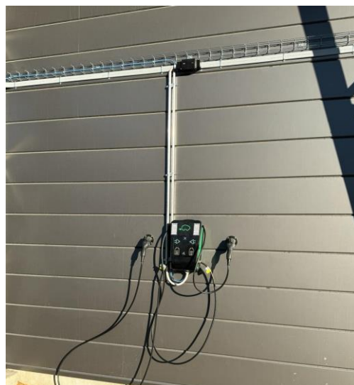
Figur 18. Ctek Chargestorm Connected 2
