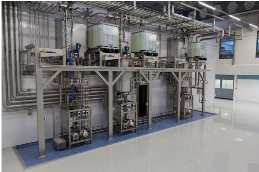
Figure 5: Process vessels and stacked raw material containers at 1st floor level in not classified basic hygiene zone as back side of Figure 5.
