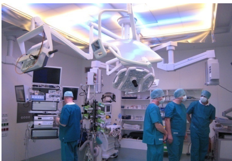
Figure 1. Operating room with UDF ceiling and installed equipment.
