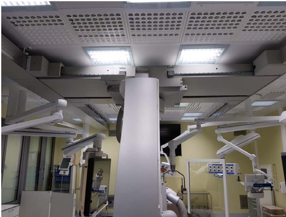
Figure 1 Hybrid Operating Room in Nya Karolinska Hospital, Stockholm, Sweden, equipped with Halton Vita OR Space 5 ventilation system
