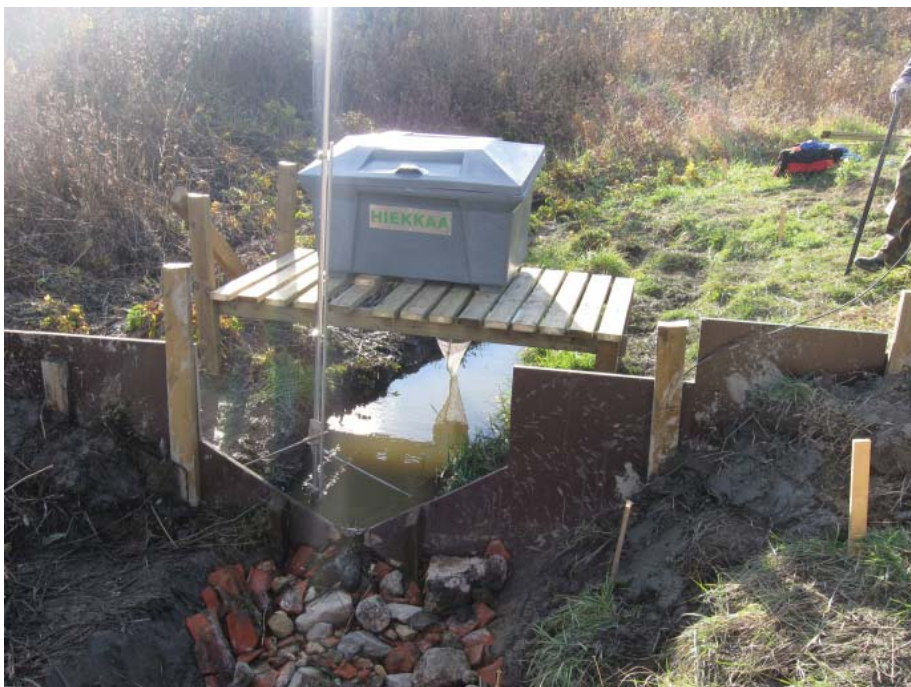
PICTURE 1. The ferric sulphate doser and the v-notch weir at Nautela. Iron chemical dissolves from a nylon netting cone at adjustable rate according to the flow conditions and precipitates phosphate from water in insoluble form. Photo: TUAS.
