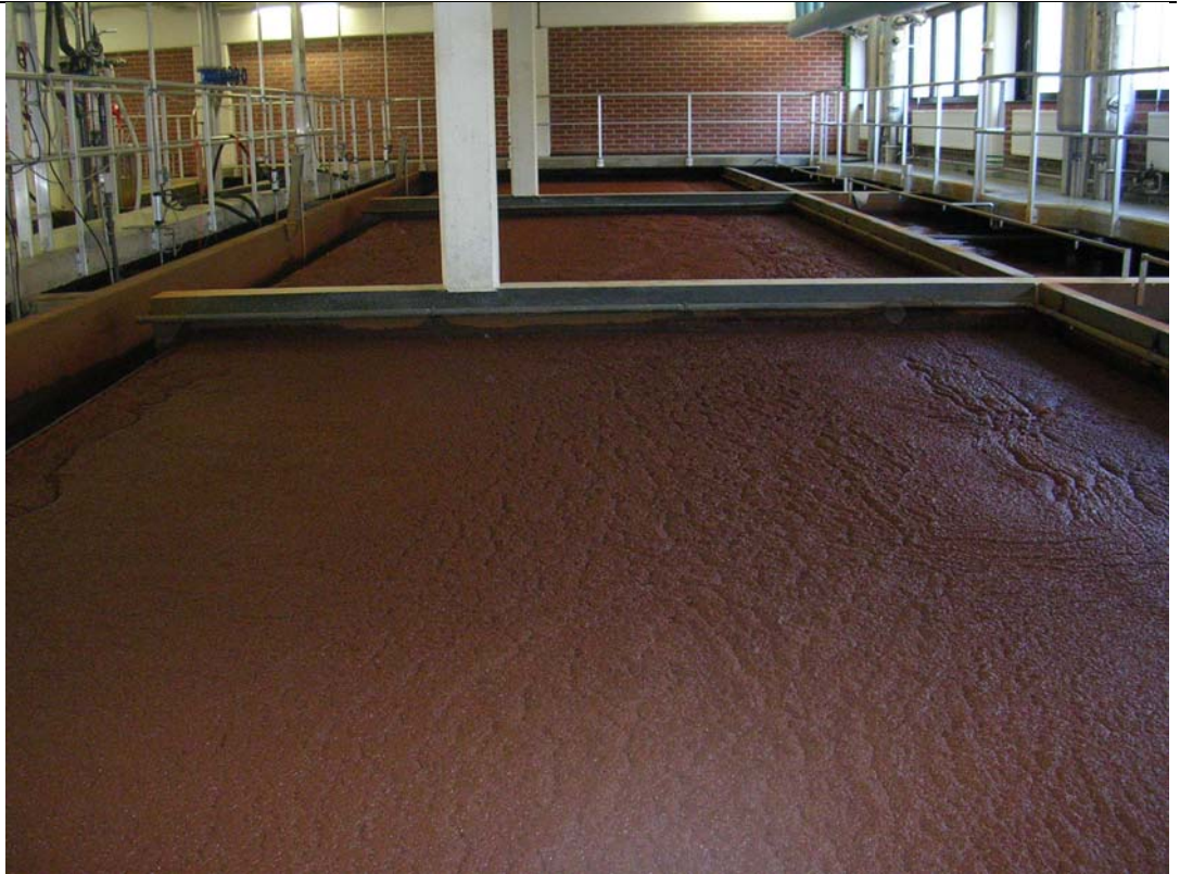
Figure 5.2. Is taken from flotation of Rusko water treatment plant, but Kämenniemi plant utilizes the same principle in smaller scale (photo by Pekka Heinonen)
