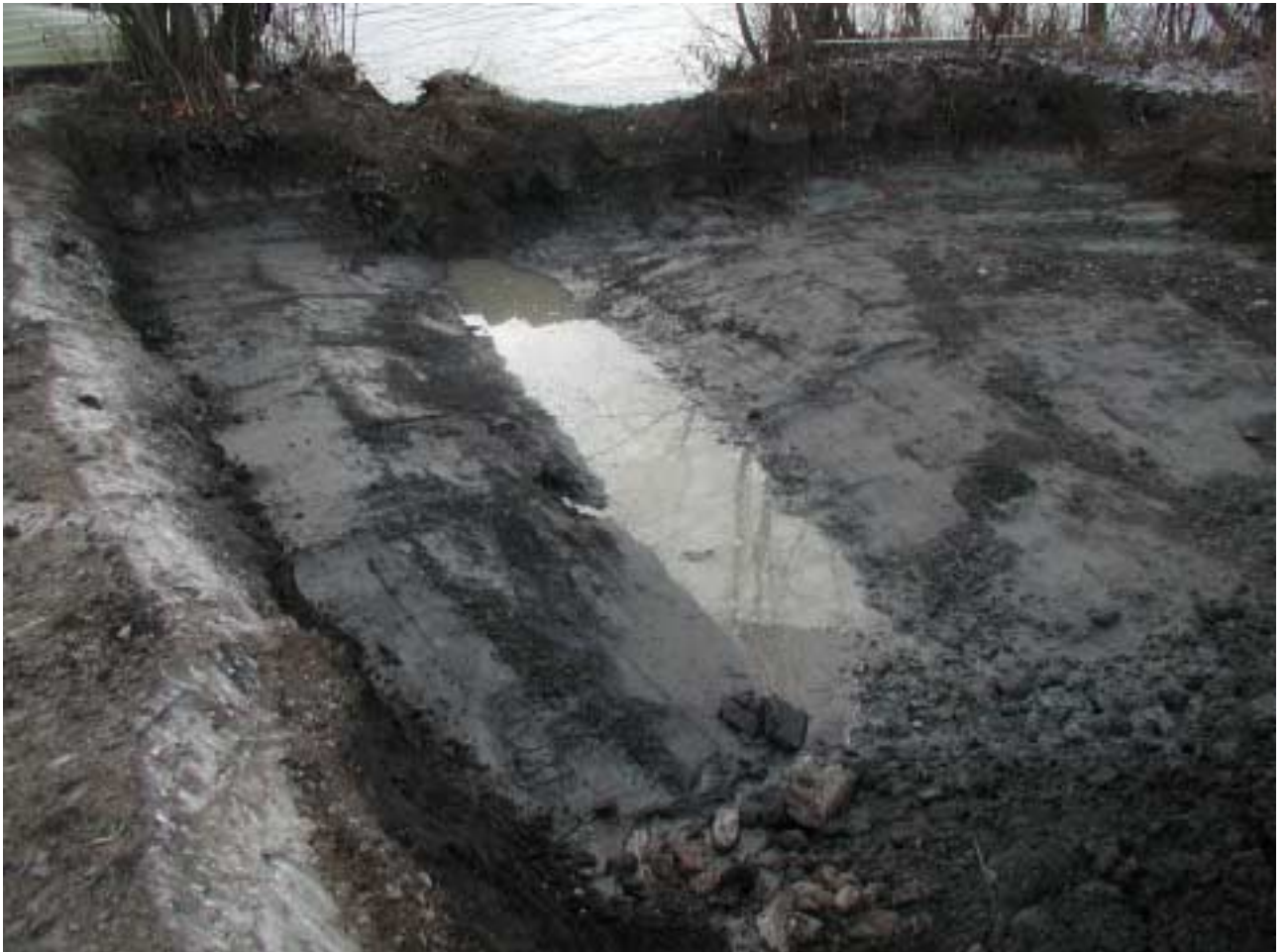
Figure 4: The mouth of the drainpipe. Drainpipe has already been removed. Orientation southwest.
