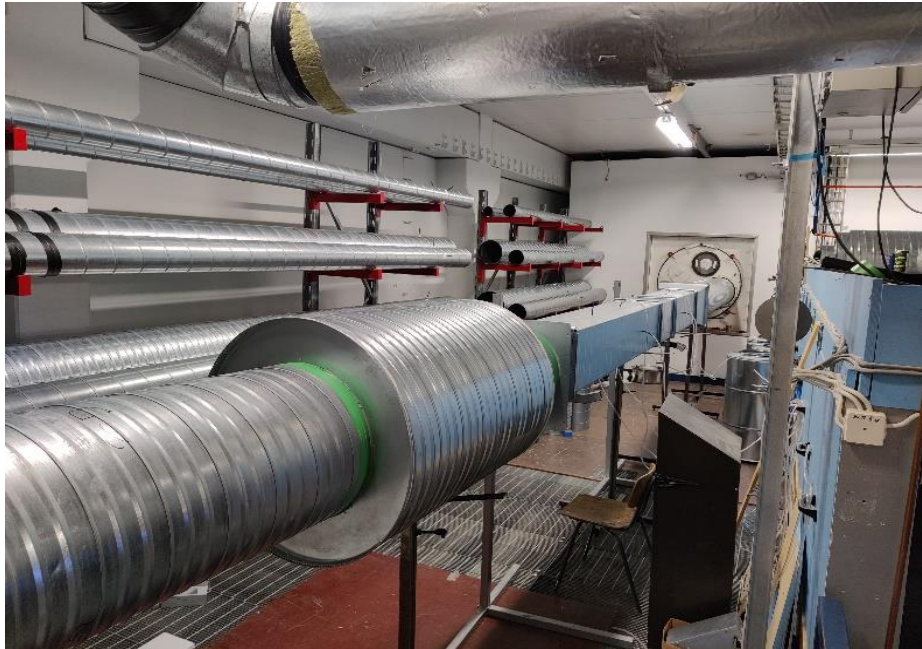
Figure 8. Installation for tests of a rectangular silencer
