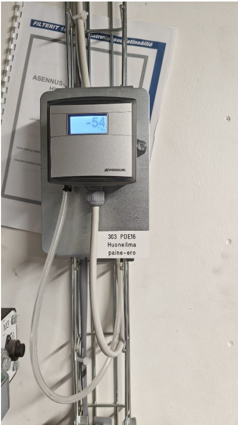
Picture 3. Example of field level device.
