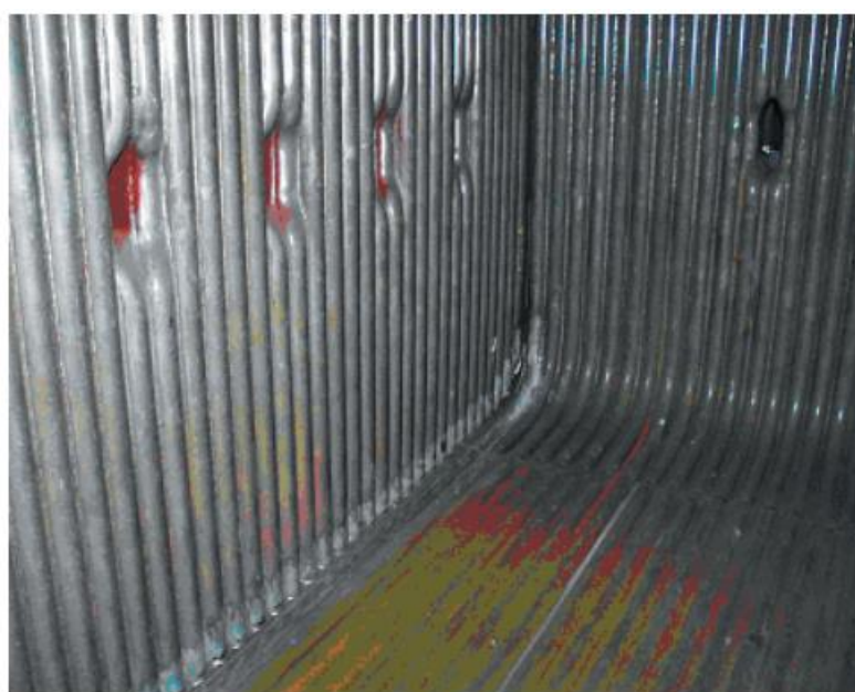
Figure 7 Carbon steel furnace bottom ( Vakkilainen, 2005, p. 10-14 )
